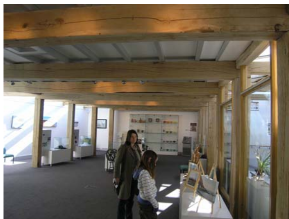
Figures: 11-13 Use of local oak felled and processed for the purpose and detailed to allow for shrinkage.
